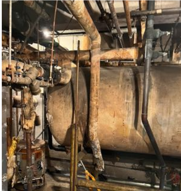
Ancient piping at boiler room
