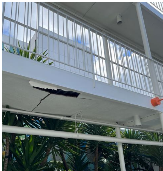
Second floor walkway on east side of property damaged by water penetration, currently offline
