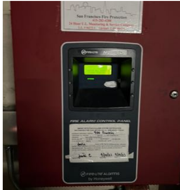
Fire alarm panel at lower garage
