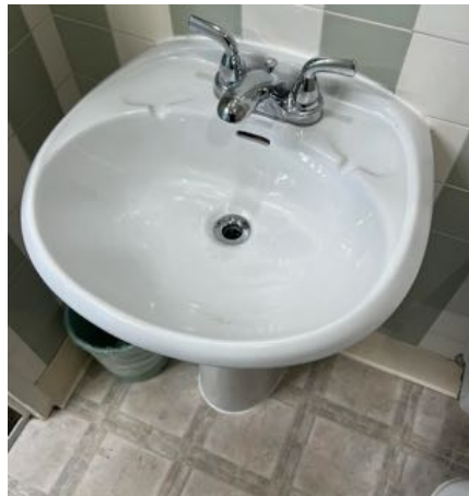
Typical bathroom pedestal sink
