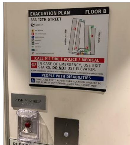
Signage and call buttons at Area of Rescue basement level
