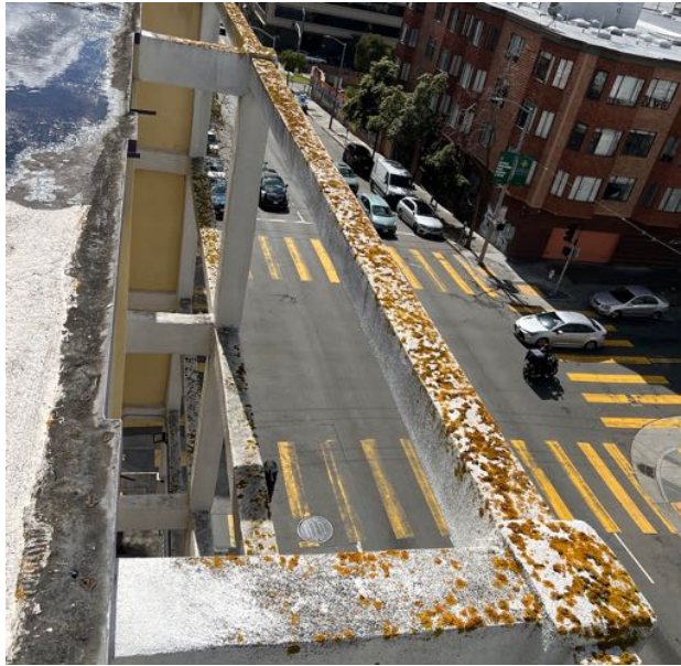
Building façade – heavy fungus
